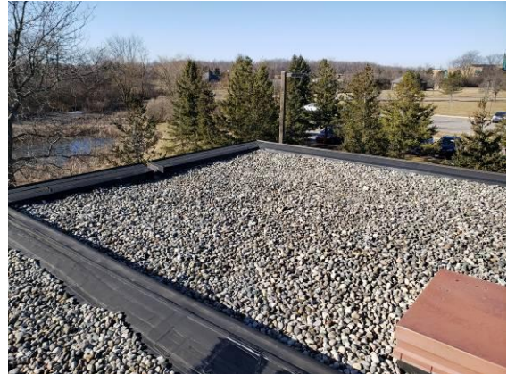
8. View of smaller south building addition, looking southwest. This roof drains to a scupper at the south wall.
