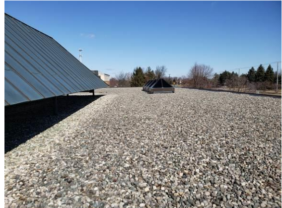
2. Another view of East Area roof, looking north. The sloped mechanical unit screen wall roof visible on left.
