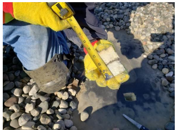
6. View of the roof core from the smaller south building addition where two layers of 1.5" foam exist.
