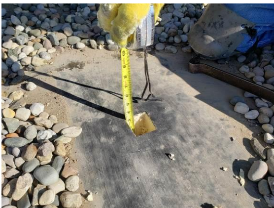
5. View of a typical core in the main roof areas. A single layer of 3" thick rigid isocyanurate foam found over a steel roof deck.
