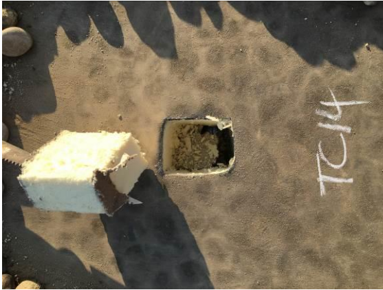
19. Photo of Test Cut #14. Insulation found dry to touch.
