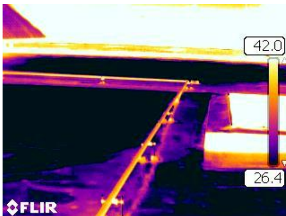
5. Image 5. One more smooth roof. No localized heat images that would be suspect of representing wet insulation. Conduits visible.
