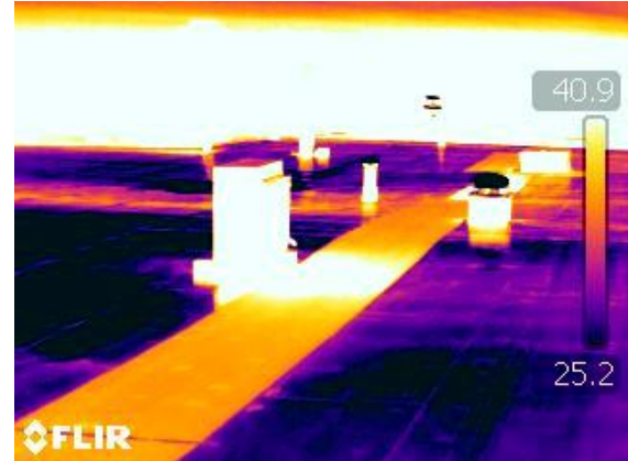
2. Image 2. Another view of the 2008 smooth roof. Walkway visible (as would be normal). Curbs and pipes also visible (as normal). No localized heat images that would be suspect of being wet insulation.
