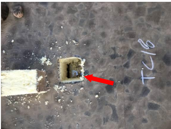
23. Photo of Test Cut #18. Insulation found dry to touch.
