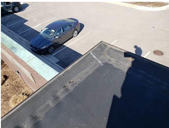
3. Holes found in the NW corner of the east area. The wood blocking at the edge visible through the holes.
