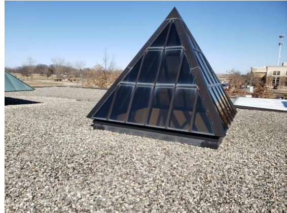
14. An existing pyramid skylight. This skylight should also be able to be reroofed without having to lift and reset the skylight and frame.
