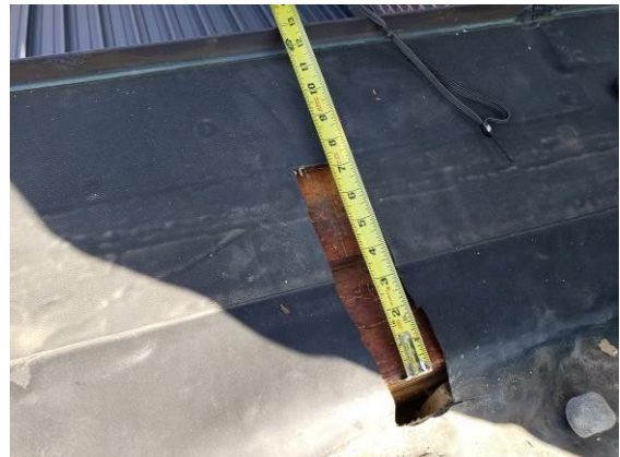
10. View of a typical raised roof edge. The wood blocking is approximately 13 inches wide and supports the EPDM roof.
