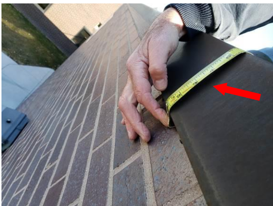
23. Close up measurement of the existing metal. Existing metal is slightly out from brick and is approximately 5 inches in face dimension.
