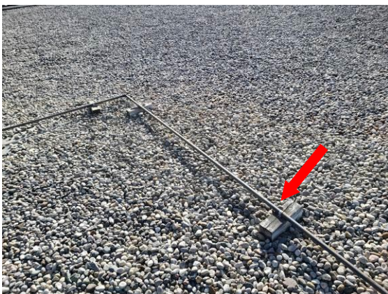
17. Another view of the existing conduit and conduit supports on the ballasted roof. With the replacement roof, newer style supports could be added that may be better systems than simple wood blocking supports.
