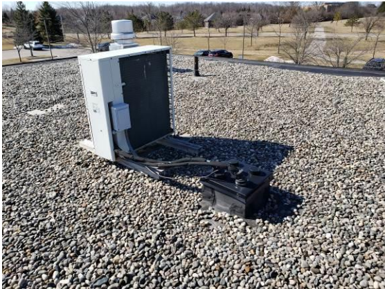
21. Localized HVAC unit on wood sleepers. Should be able to be raised a few inches to sit on newer sleepers and pads with the new roof system.
