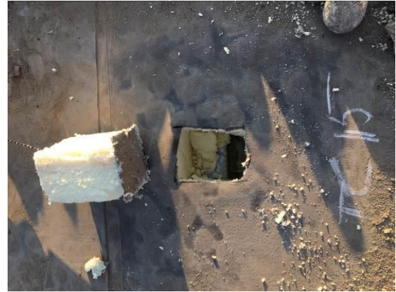
20. Photo of Test Cut #15. Insulation found dry to touch.
