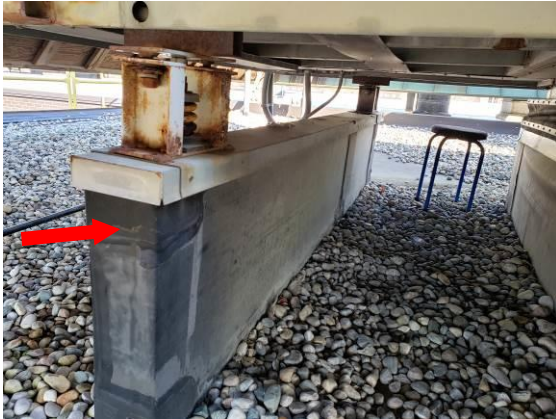
13. View of equipment sleeper supports. Reroofing should be possible without having to lift the large units.
