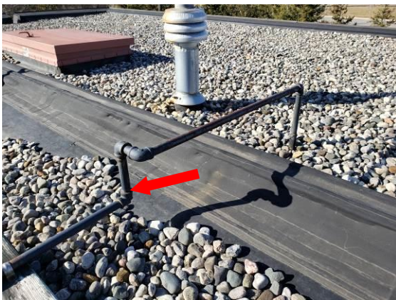
15. Most gas and/or electrical conduit is high enough to remain. Some areas may have to be lifted, depending on the thickness of the recovery insulation.
