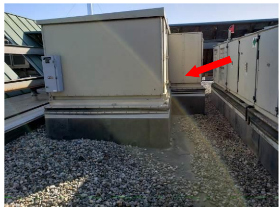
12. Another view of large rooftop penetrations and some limited spacing between the units.
