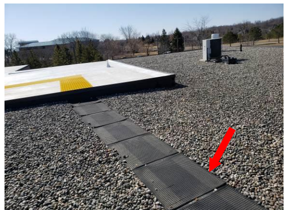
24. Typical existing walk pads. With replacement roof new safety yellow walk pads could be installed, similar to those installed in 2008.
