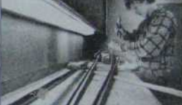
Electrician Patty Durand installs strip electrical conduits in a library study room.
